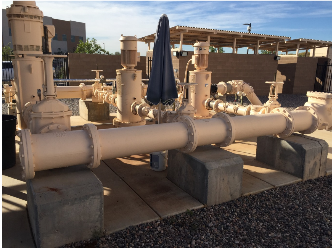
Figure 1.3 Health Center Water Production Facility Booster Pump Station
